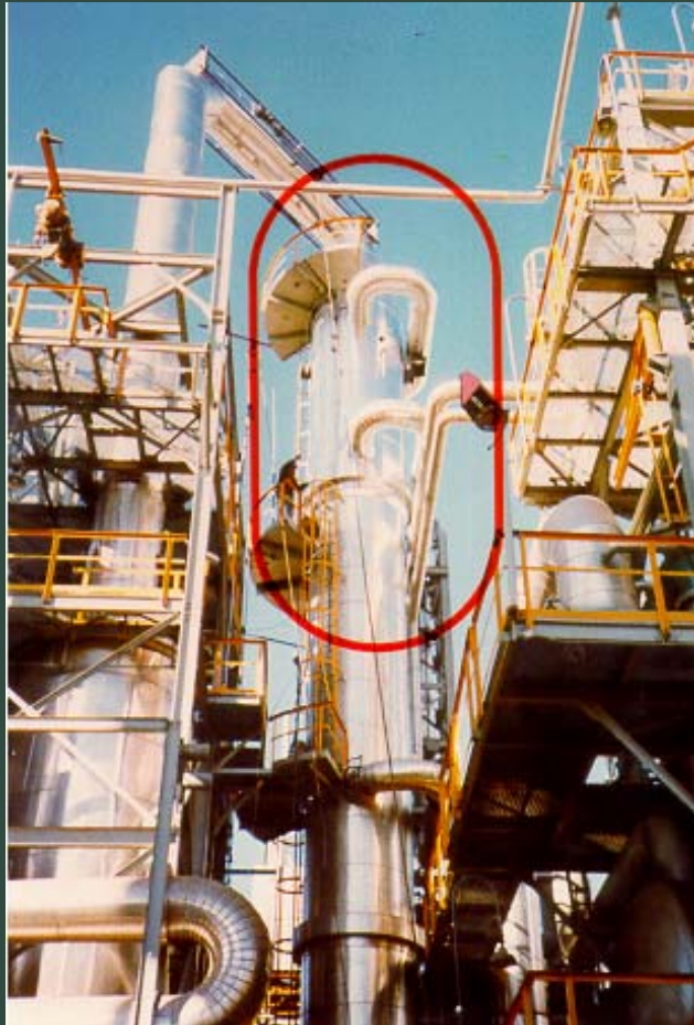
Reactor of a Feed vaporizer plant
